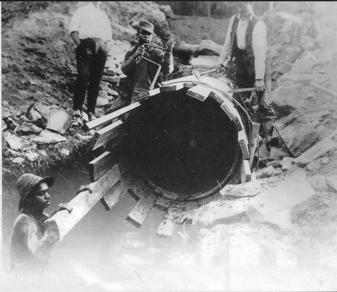
With little opportunity for job training, most African Americans a century ago could only find work as unskilled laborers, such as those photographed laying pipe in Philadelphia.
